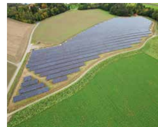
› Ground-mounted system Kraiburg approx. 13 MWp
