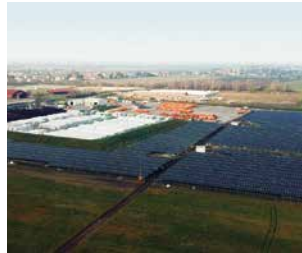
› Ground-mounted system Wien approx. 112 MWp
