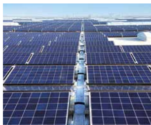
› Rooftop system Frankenthal approx. 14 MWp
