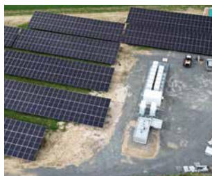
› Ground-mounted system Rote Jahne Doberschütz approx. 6 MWp
