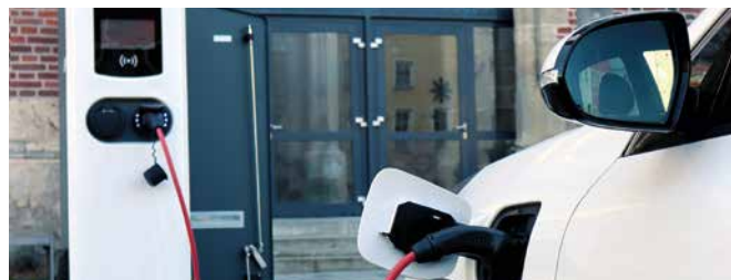
› Largest charging park in the Traunstein district 10 AC charging points 2 DC charging points
