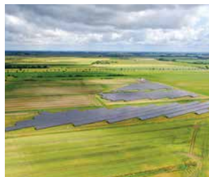
› Ground-mounted system Lehe approx. 14 MWp
